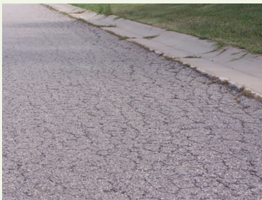
Figure 4 This pavement remains incomplete. The surface layer was never built, even after all of the subdivision lots were developed.
