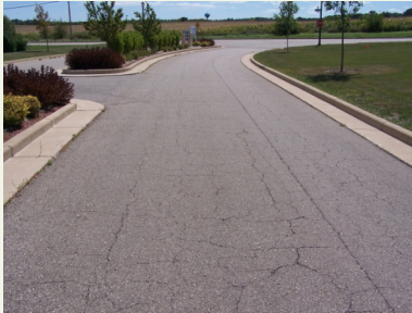
Figure 3 A binder layer showing fatigue distress, which results from a first-stage pavement structure that is underdesigned for the loading conditions
