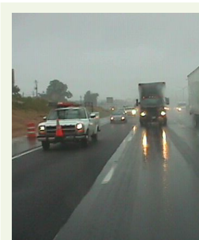
Figure 6 The open graded friction course shown in the left lane reduces standing water and pavement noise. (Image courtesy of Asphalt Pavement Alliance)
