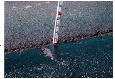
Overlays can be very thin and still add structural support and years to a pavement’s life. (Image courtesy of APAM)
