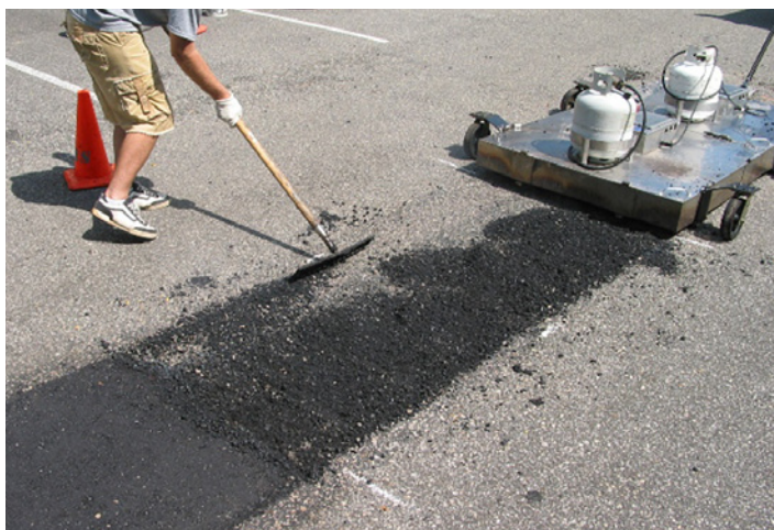
Prevent a small problem from becoming a big one. (Image courtesy of Asphalt Reheat Systems, LLC)
